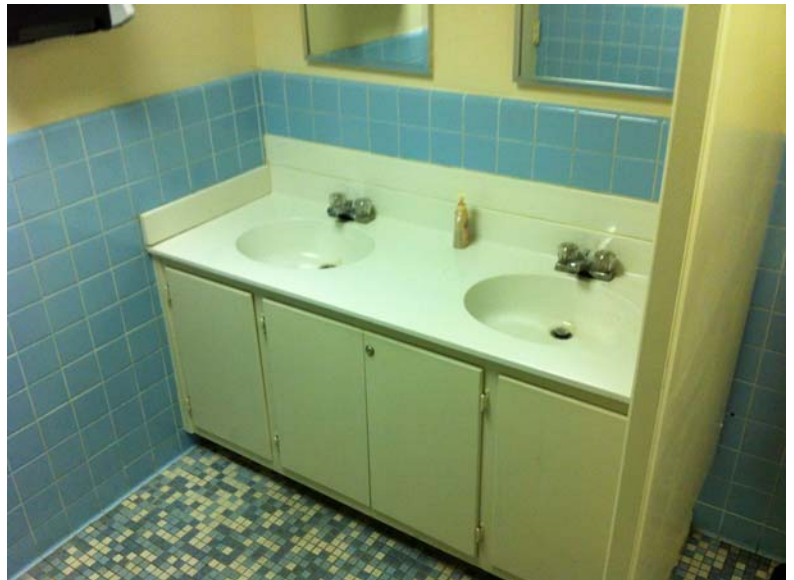
Picture #2 – The current sinks in all public bathrooms do not allow the ADA required clearances below the sink, proper height, and the proper grips on the faucets.
