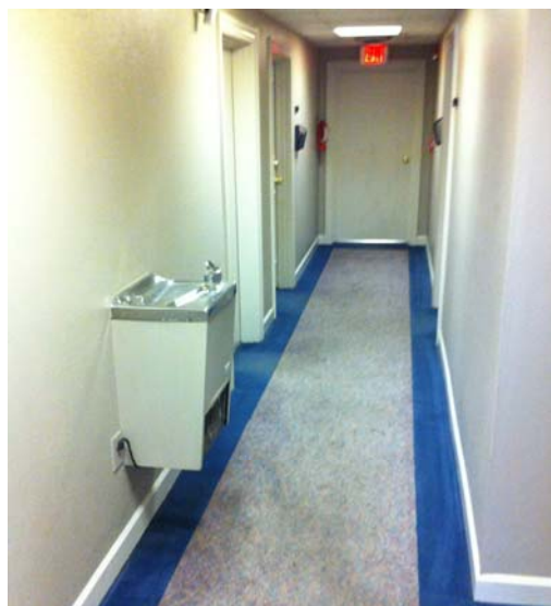
Picture #3 & #4 – The typical Water Fountain location at all three levels do not provide the ADA required height, clearance under fixture or room to allow required approach distance. The fixtures also create a protruding object within the accessible path by more than 4 inches without cane detection. In addition, the fixtures block the emergence egress path.
