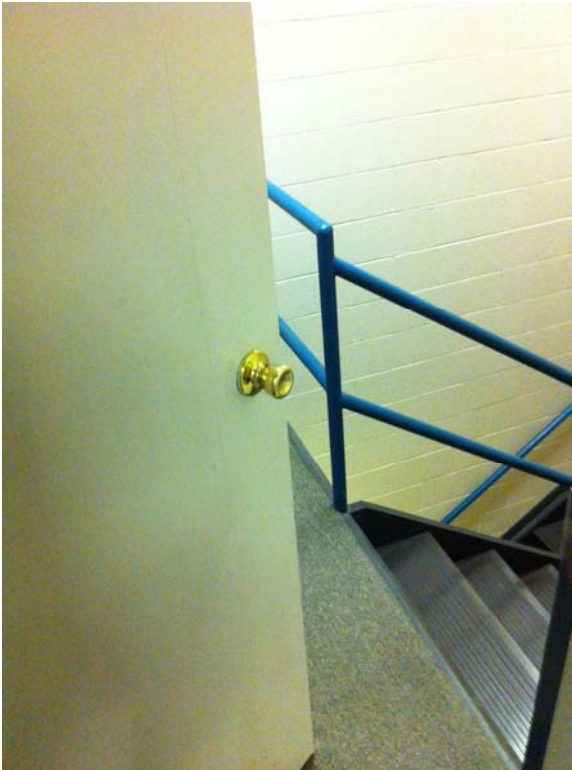
Picture #5 Non-compliant door hardware
